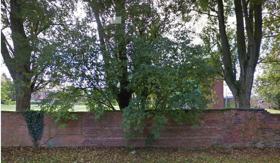
Boundary wall and trees looking south towards the northern gable end of the Mayfield building
